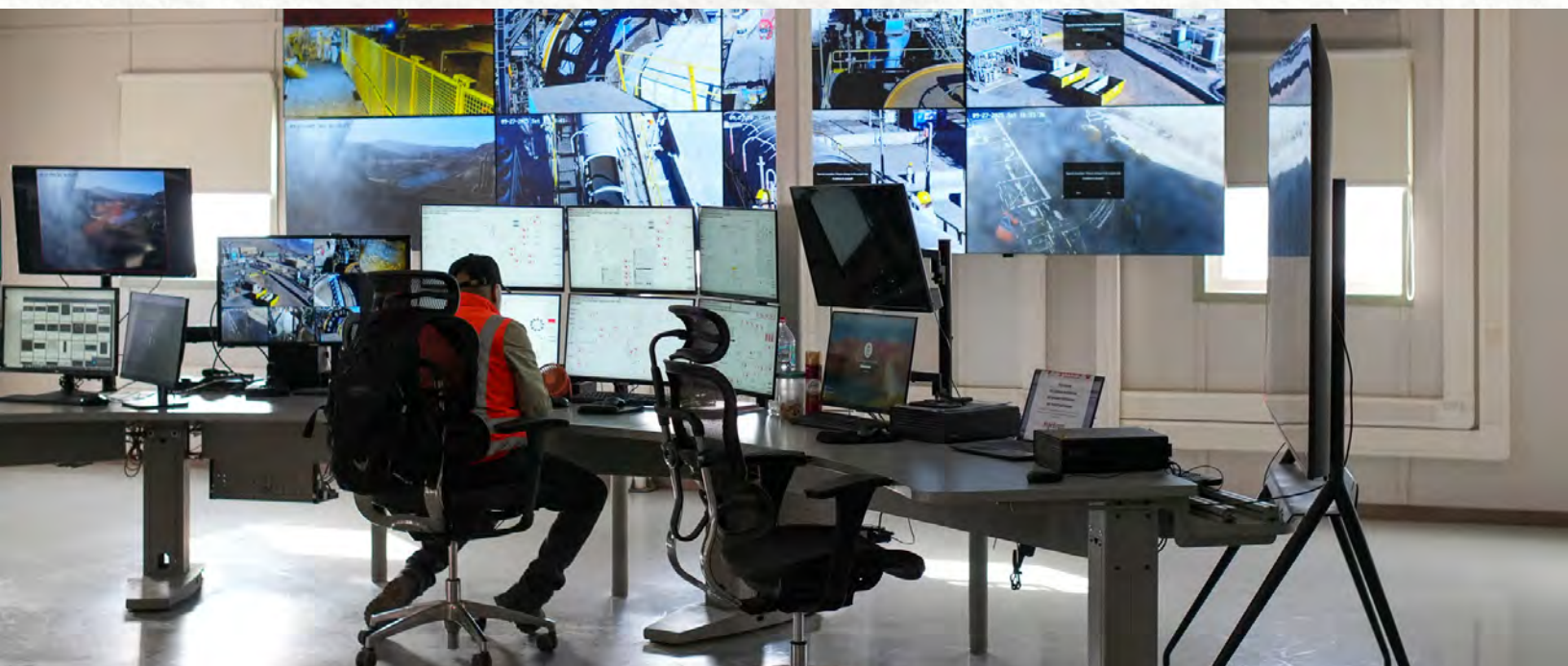
Mantoverde – Concentrate Plant Control Room
