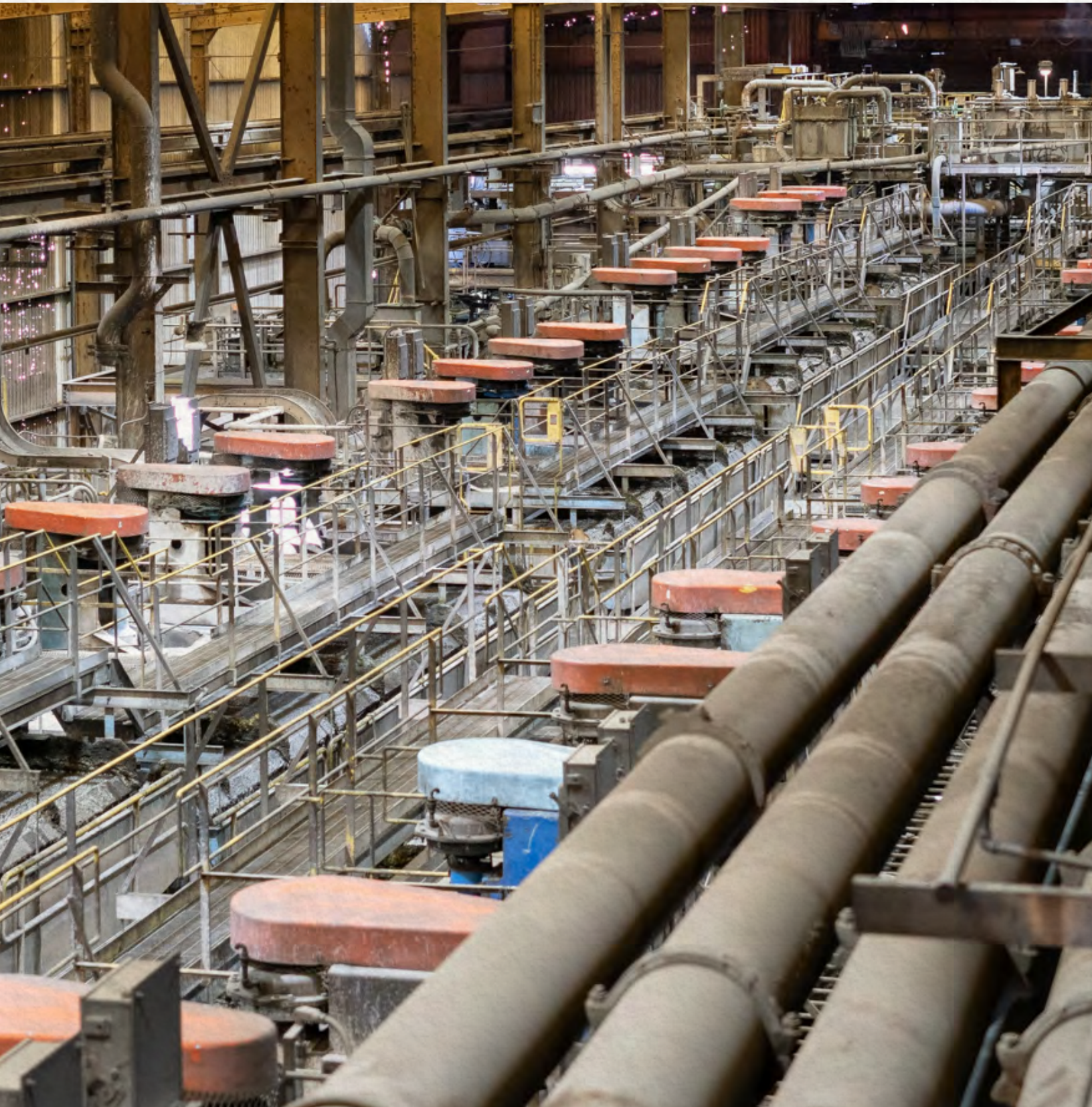
Pinto Valley – SX/EW Plant
