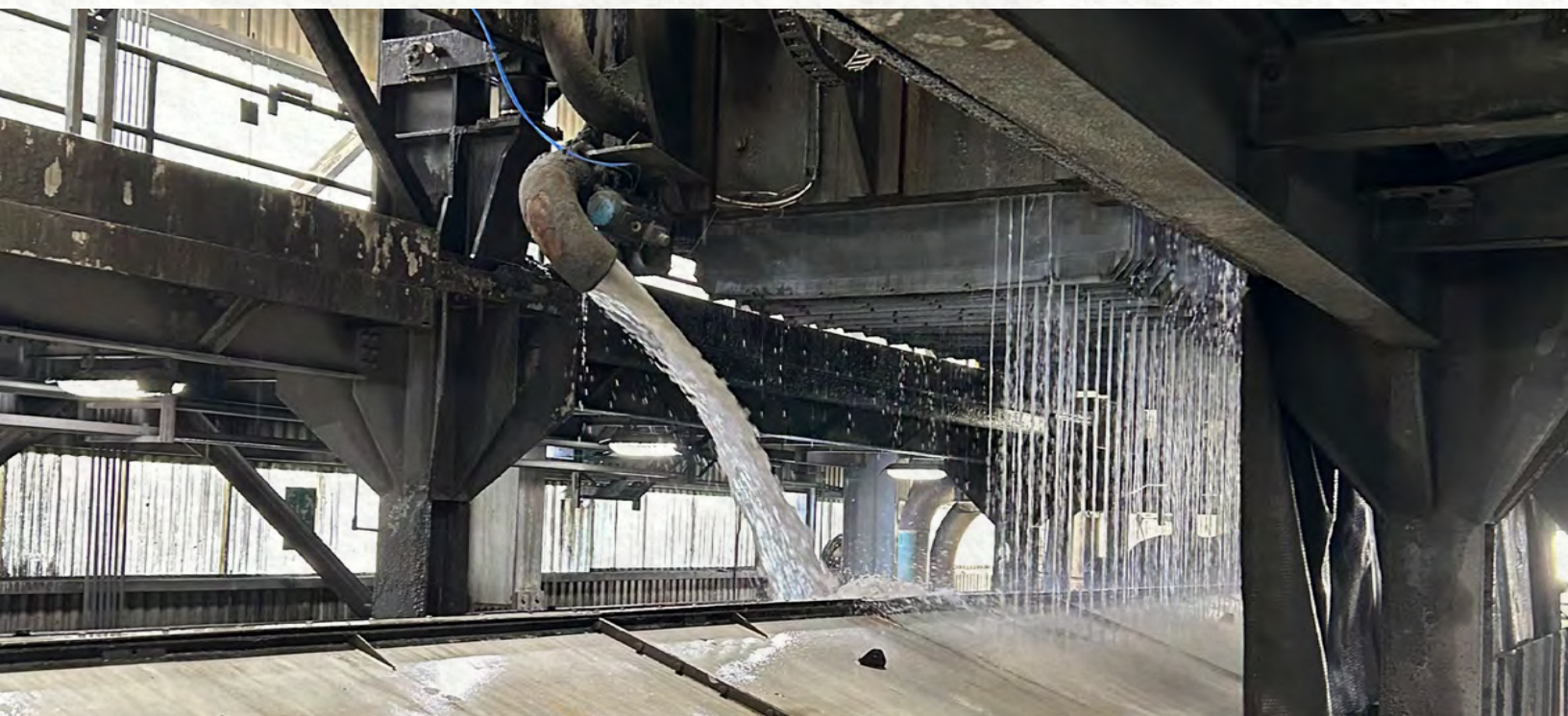
Cozamin - Water Recovery in Dry Stack Plant
