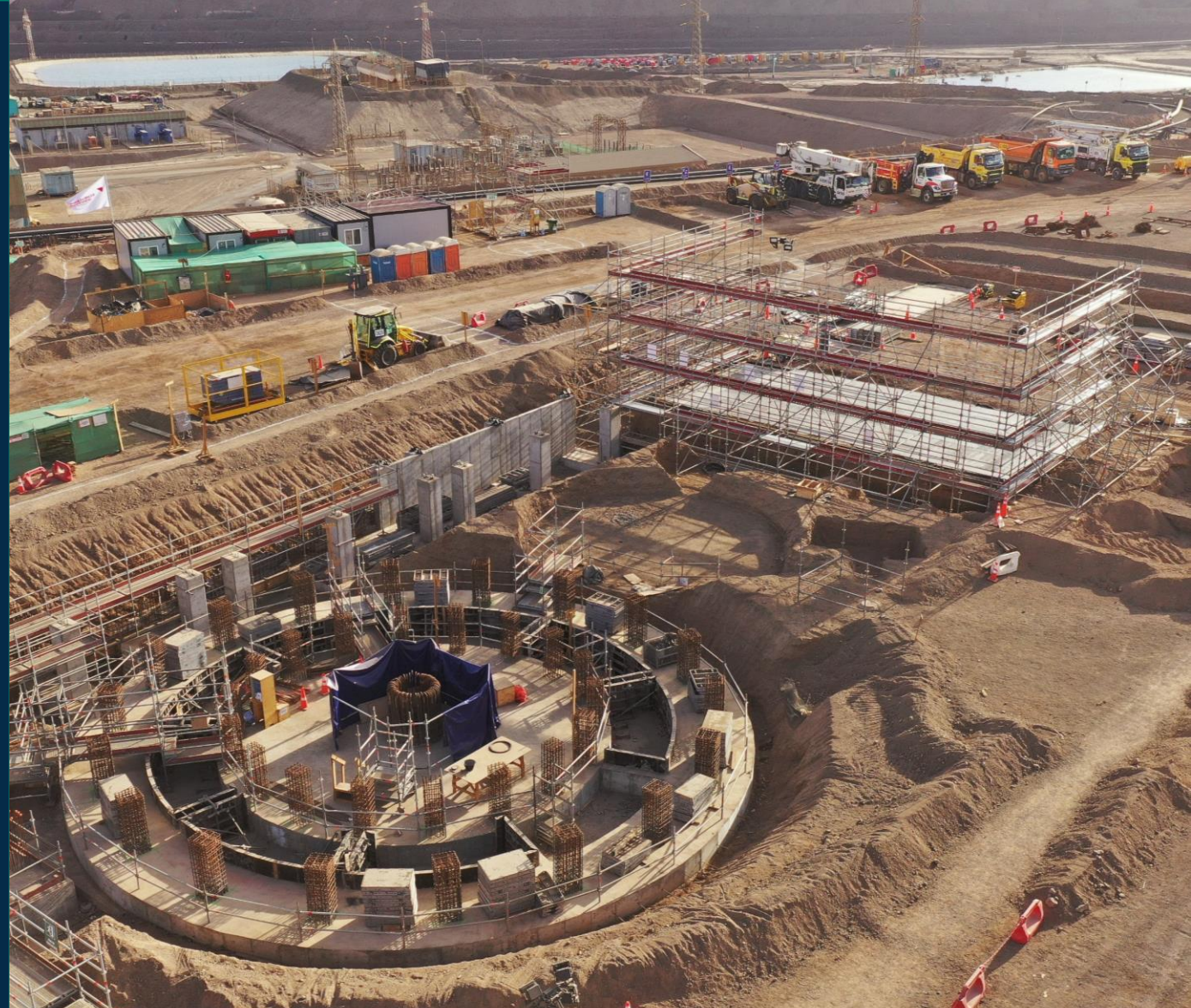
Photo: Mantoverde Development Project ("MVDP") Cu Thickener and Filtration
