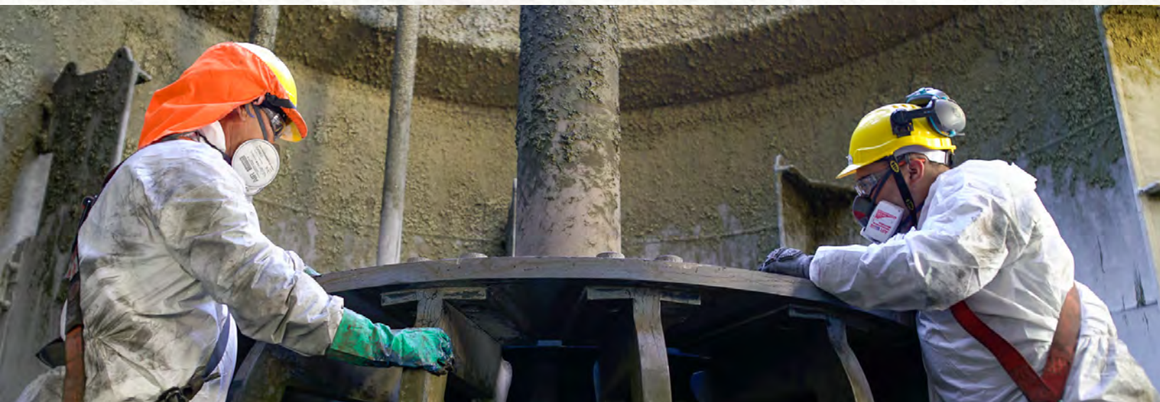
Mantoverde – Plant Maintenance
