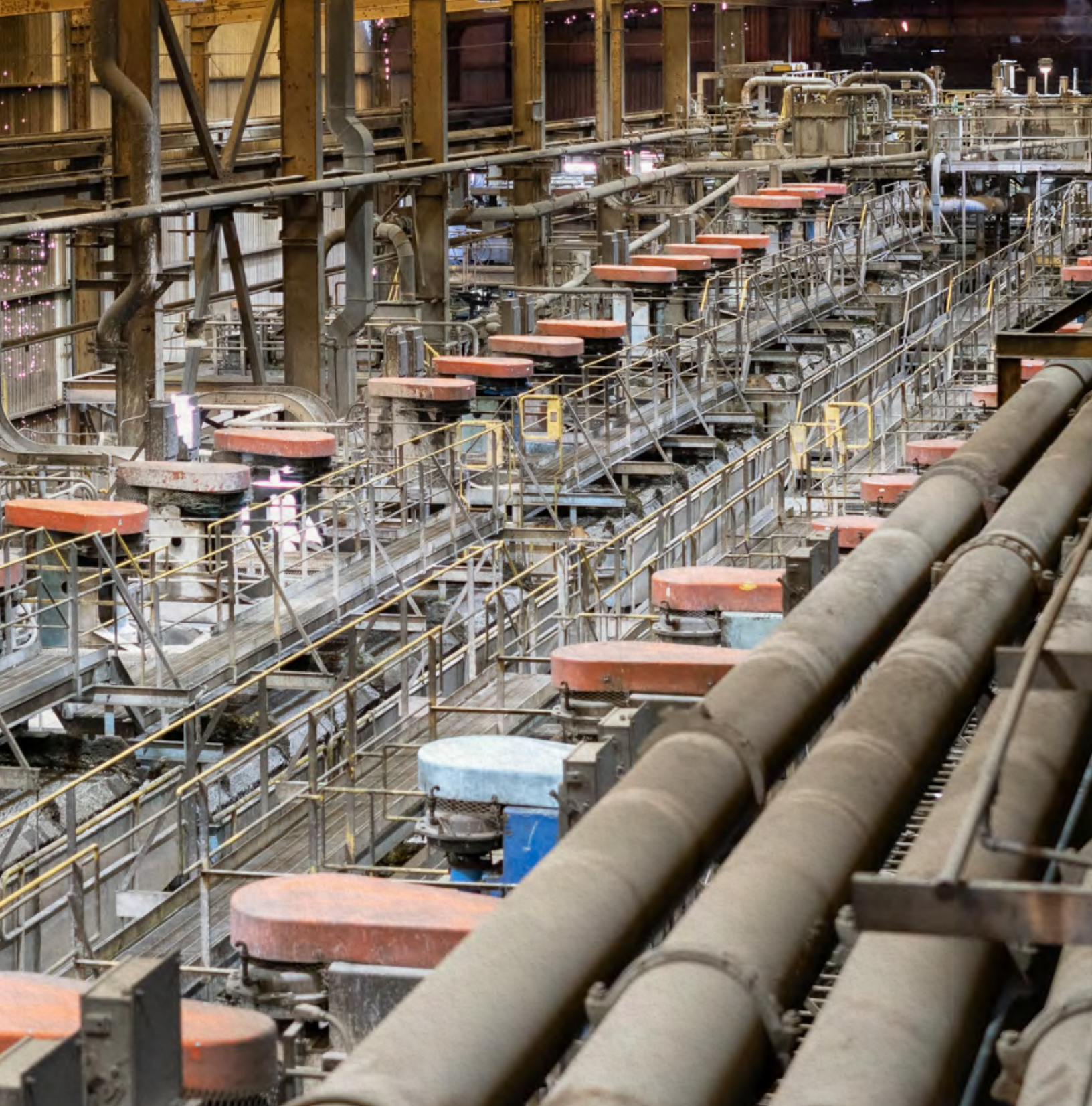
Pinto Valley - SX/EW Plant
