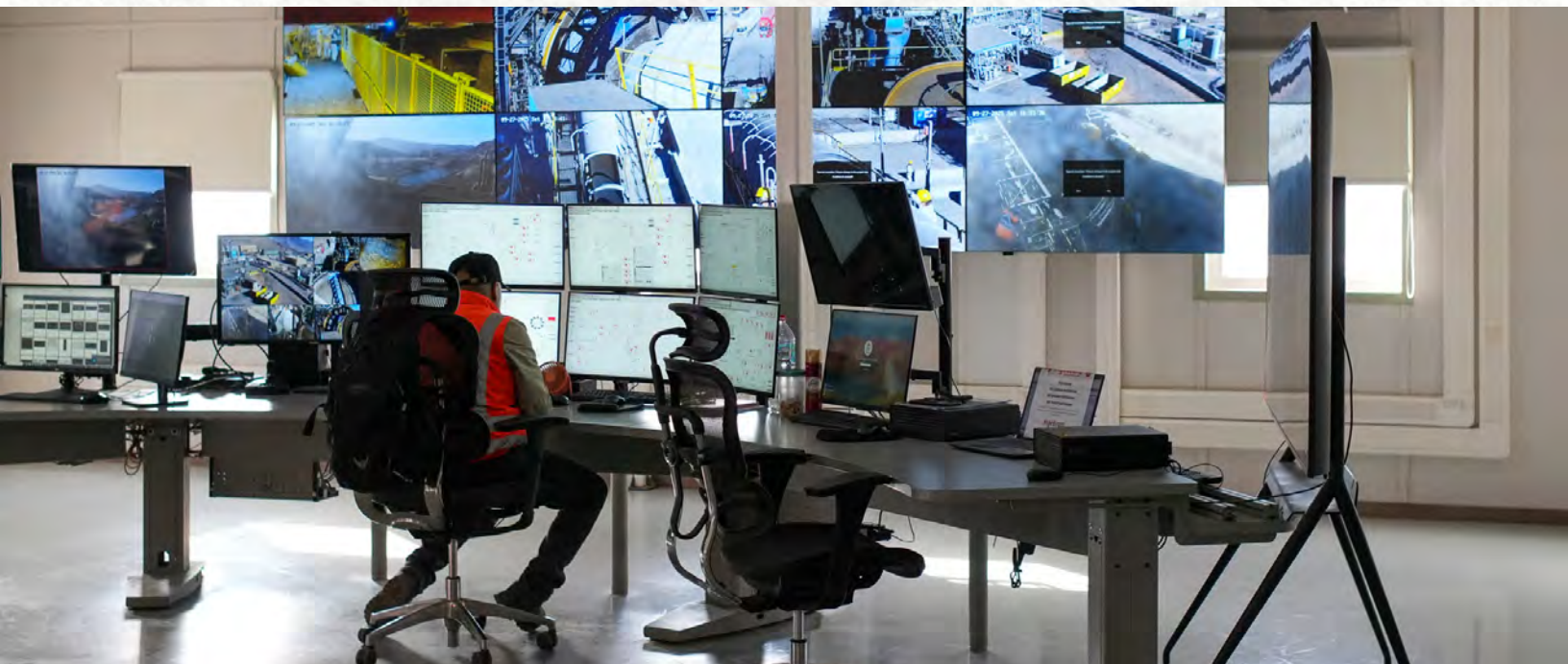
Mantoverde – Concentrate Plant Control Room
